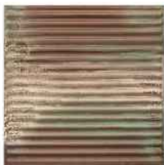
261 - Corroded Metal (V1)
