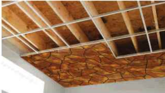
Deconyx panels supported with wooden frame structure
